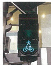
Figure 2. Example of a combined pedestrian and bicycle lantern
